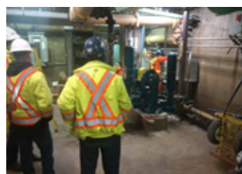
HPE Series Belt filter press feed pumps for primary sludge transfer
