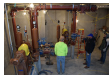
PE Series WWTP expansion, new digester recirculation pumps
